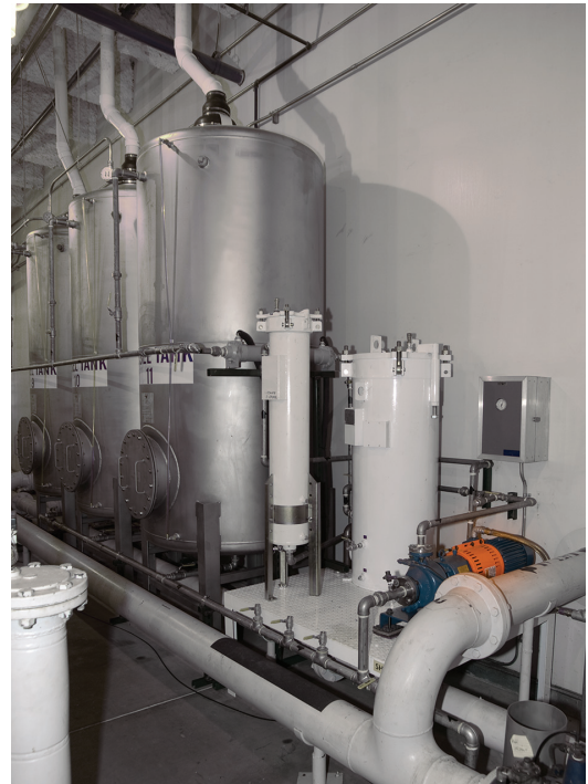
Diesel Storage Tanks
